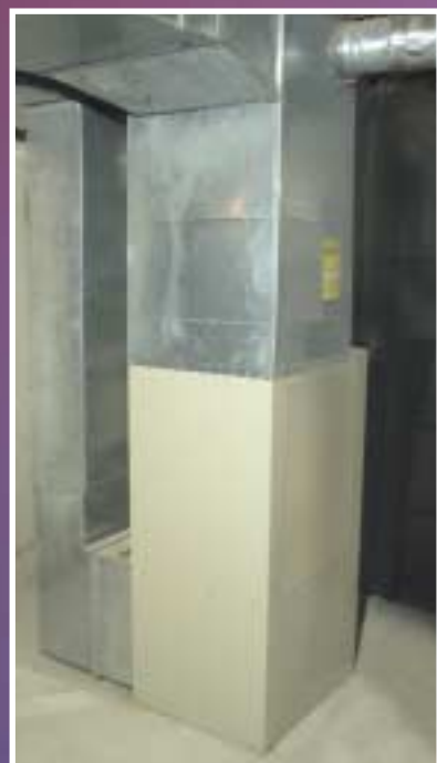
Hydro-air and heat pump backup
